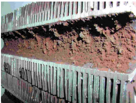
Oxygen Pitting Requiring Tube Replacement
