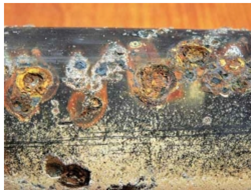
Oxygen Pitting Requiring Tube Replacement
