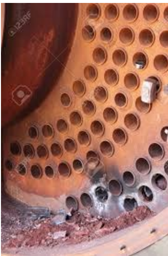
Leaking Firetube Boiler
